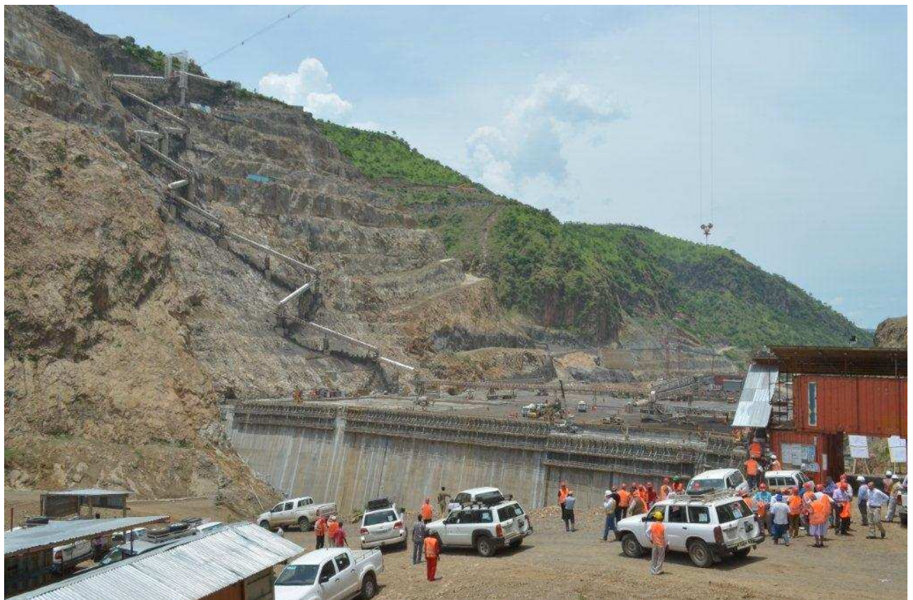
GIBE III Dam under construction (246 m high RCC dam for 1 870 MW Hydropower)
